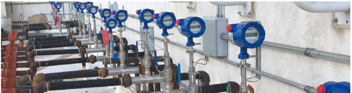
FT1 meters installed for natural gas sub-metering at a major hotel/casino in Las Vegas, NV.
