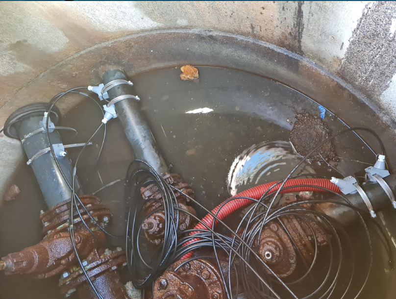
Three pairs of ultrasonic Clamp-on flow sensors installed on water pipes
